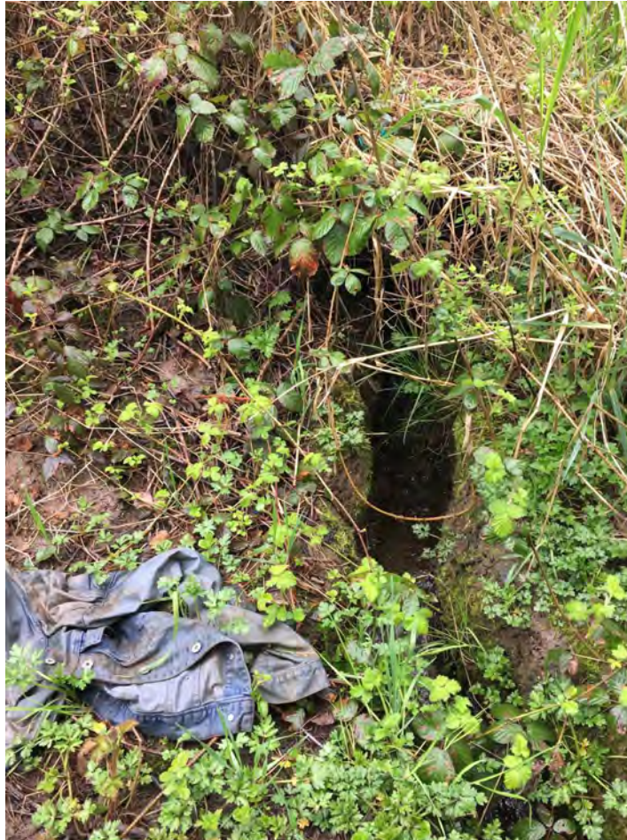
Figure 5. Eroded channel from pipeline next to littered clothing.
