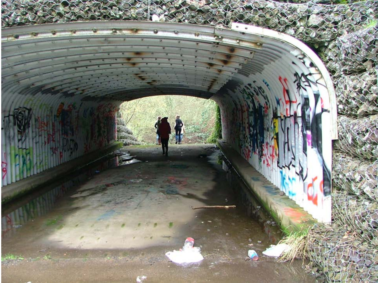
Figure 2.7 Eastern overflow culvert at end of the Cozine Creek property underneath berm. Photograph by Professor William Fleeger 2016.
